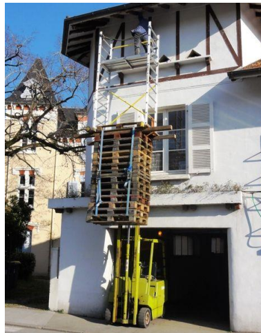
Figure 4 Working at Height Permit
